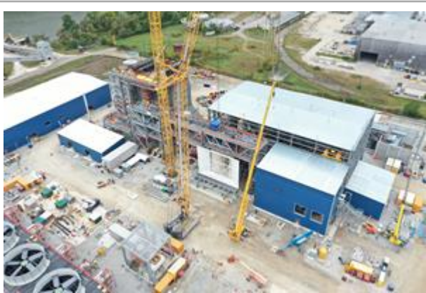
Long Ridge power plant under construction in Hannibal, Ohio. Photo courtesy of Kiewit.
